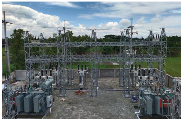
Installed 132/33kV Substation at Comilla
